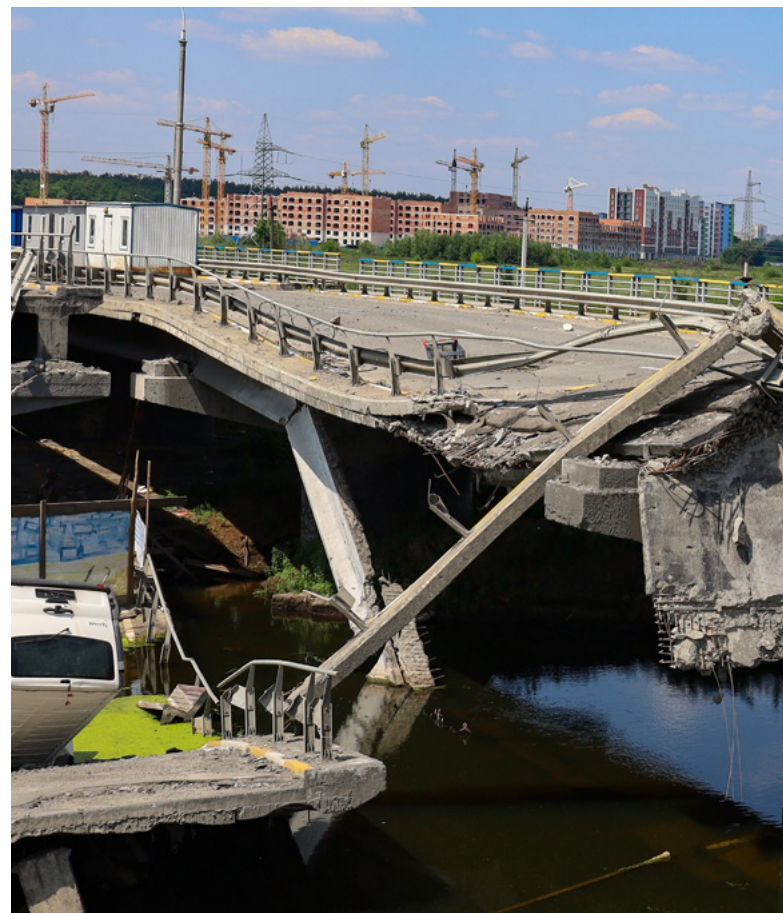
A war-damaged bridge in Ukraine. © Oleksandr Polonskyi/Shutterstock.com, 2022
